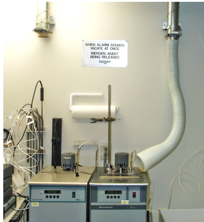
Figure 1 Ventilation system for removing oil vapors.
